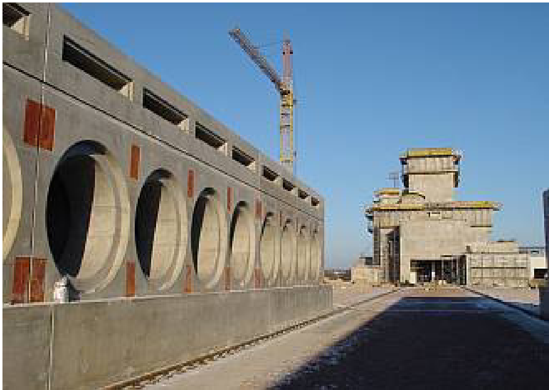
Fig. 5.34. ISF-2 storage modules.
